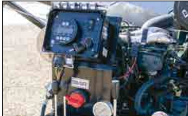
Fig 11 - Diesel engine control box
