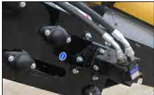
Fig 61 - Conveyor belt hydraulic drive motor
